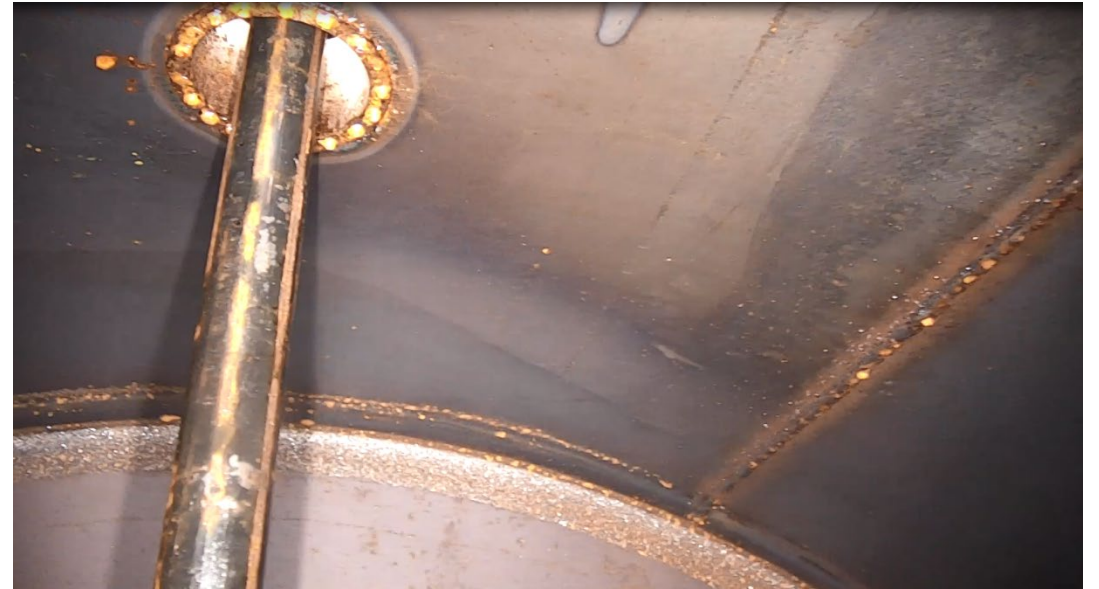
Corrosion in fuel tank to be replaced
