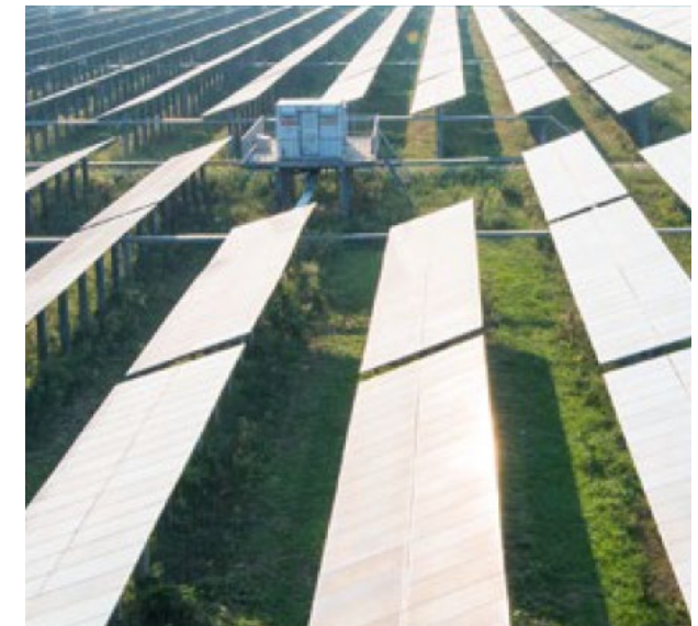
Example of a solar array
