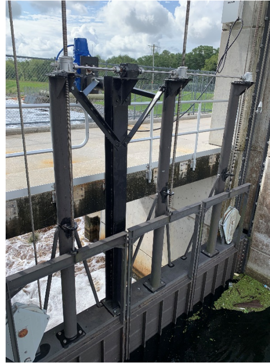
Motorized actuator connected to the gate
