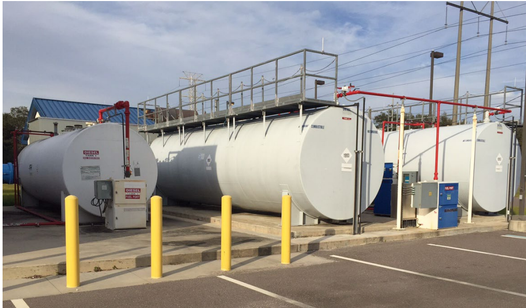
High Service Pump Station diesel fuel tanks
