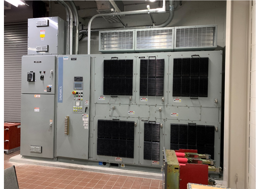
Variable Frequency Drive and Breaker
