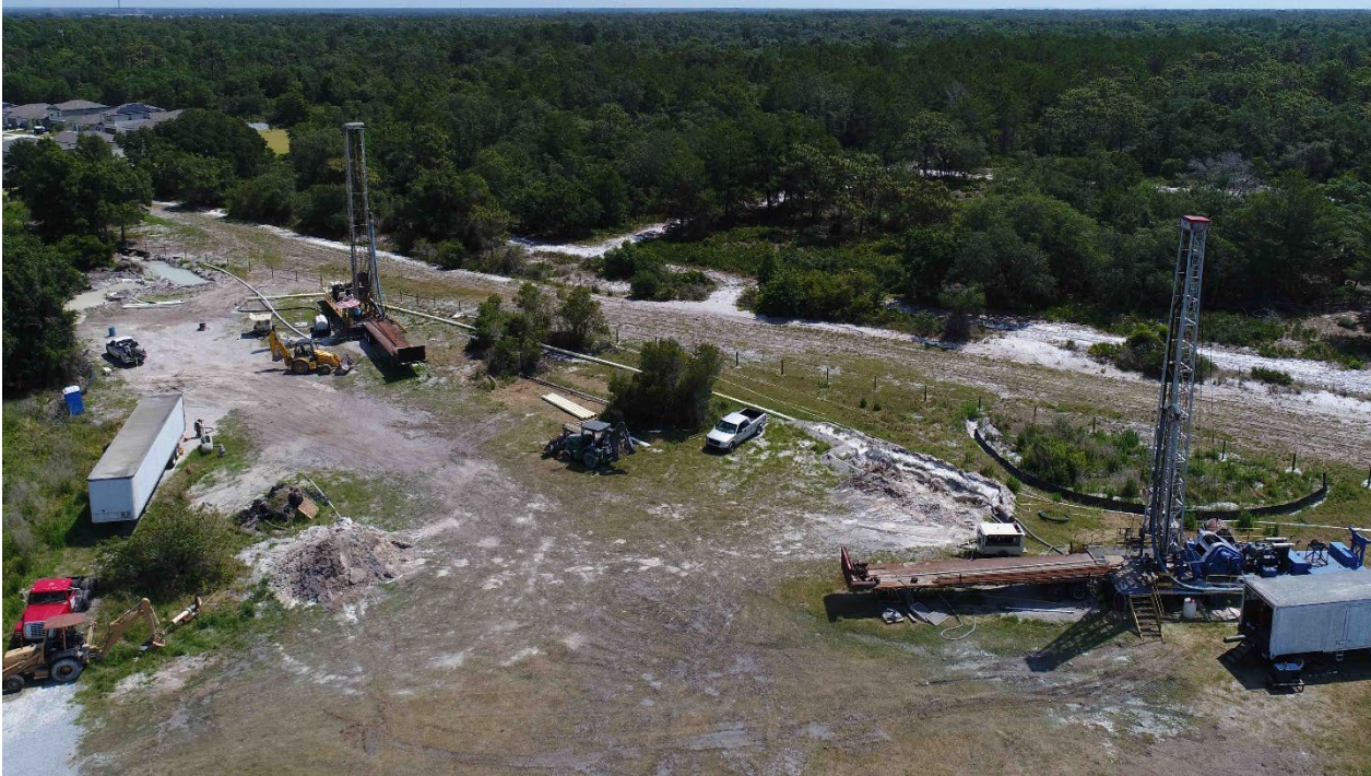
Drill rigs set up for the test well and a monitor well
