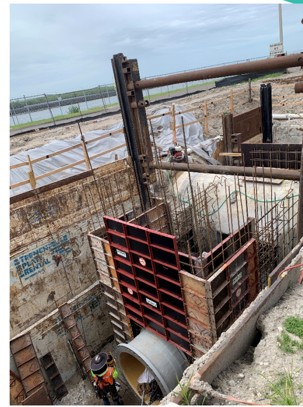
Manhole for valve and 54" stub-out pipe
