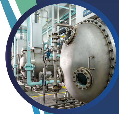
HYDROGEN SULFIDE REMOVAL
